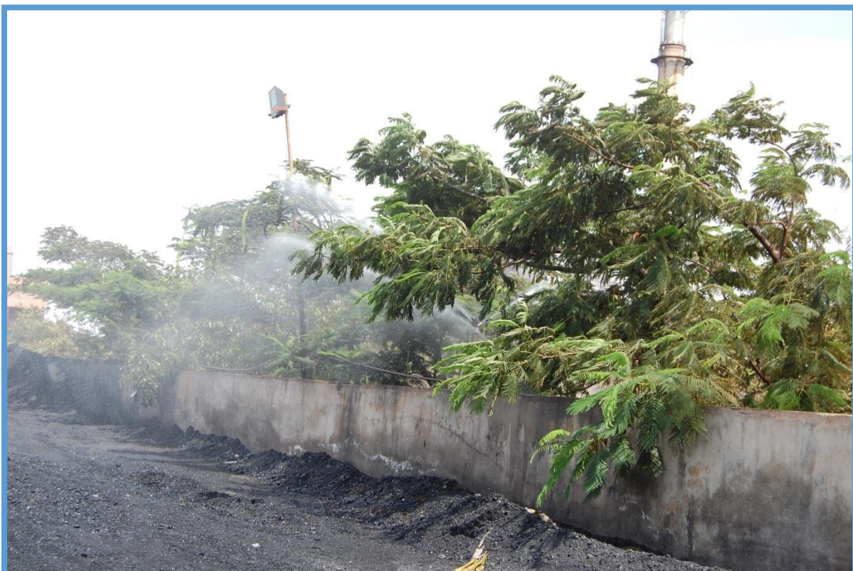
Sprinklers Installed at Coal Yard
