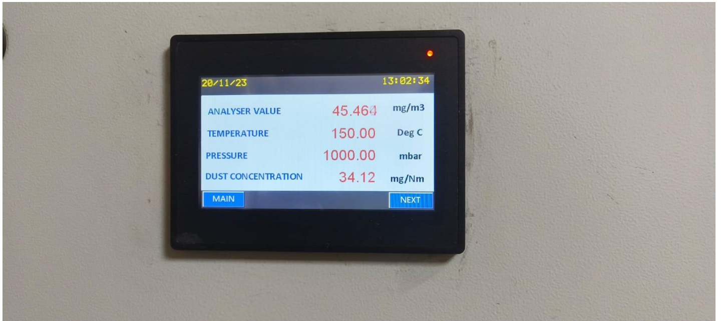
OCEMS display unit installed in our plant
