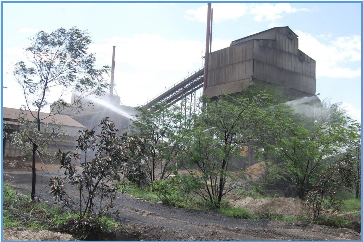
Sprinklers Installed at Bottom Ash Handling Area
