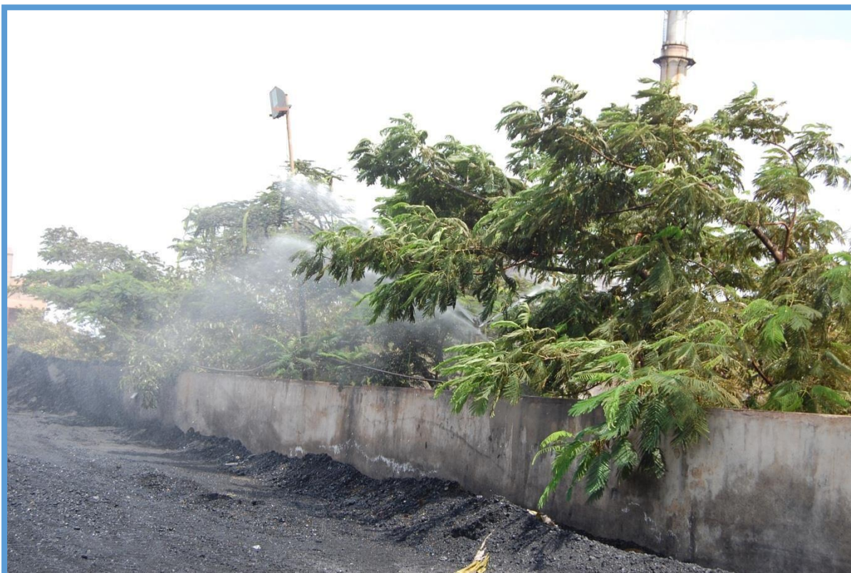
Sprinklers Installed at Coal Yard
