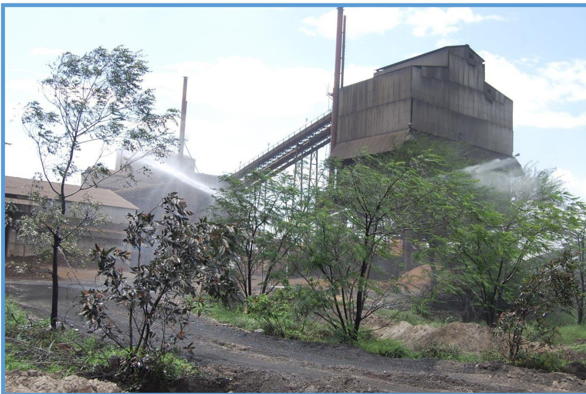
Sprinklers Installed at Bottom Ash Handling Area
