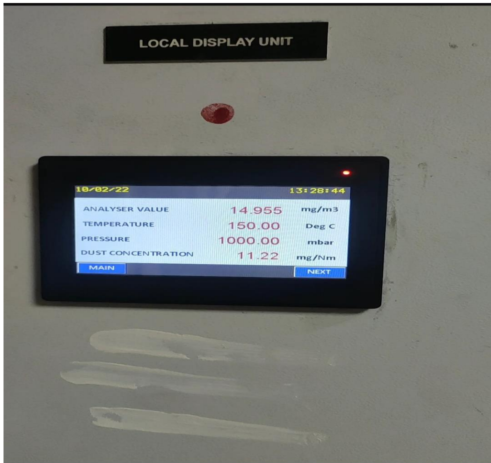
OCEMS display unit installed in our plant
