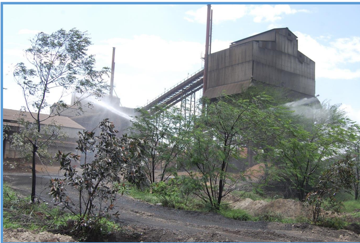
Sprinklers Installed at Bottom Ash Handling Area
