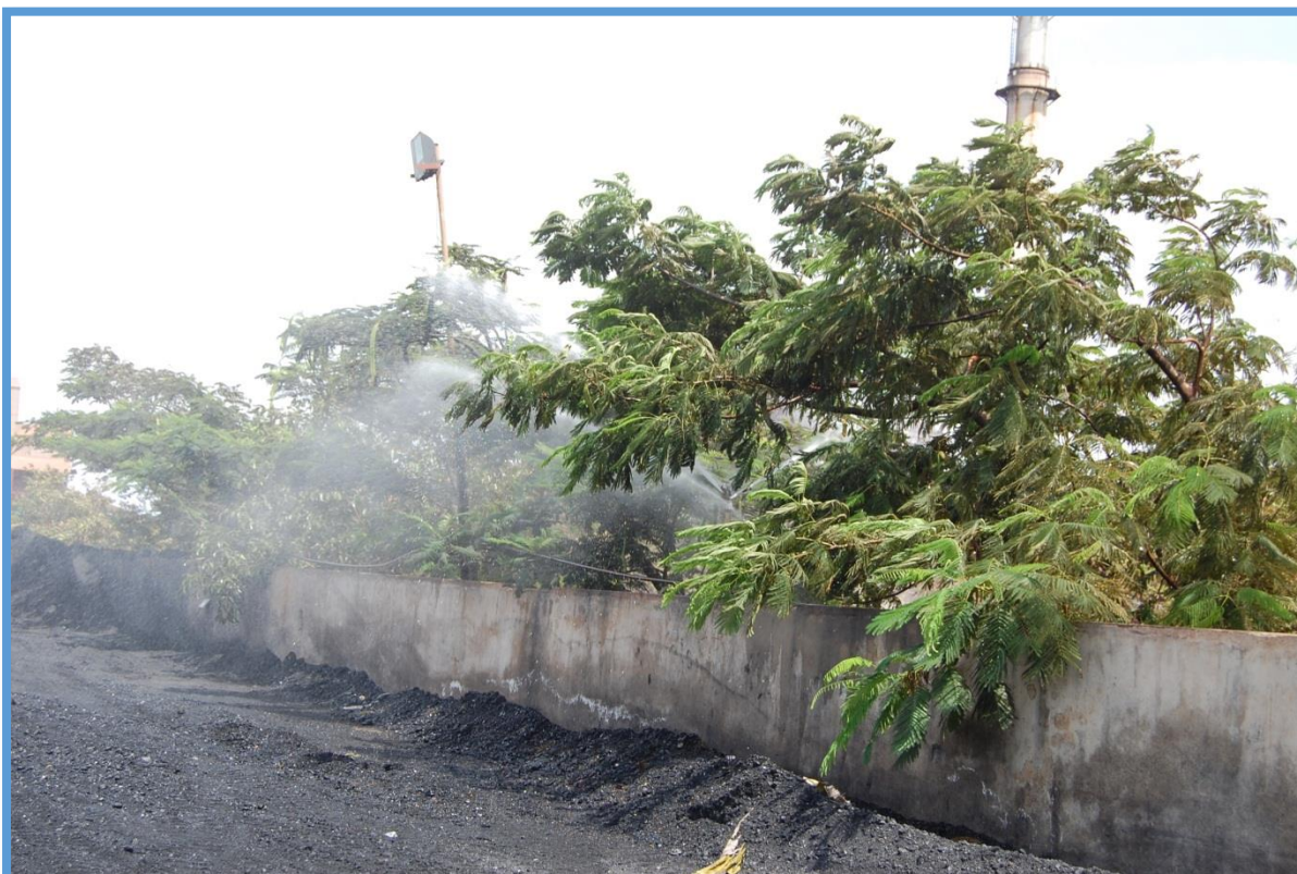
Sprinklers Installed at Coal Yard
