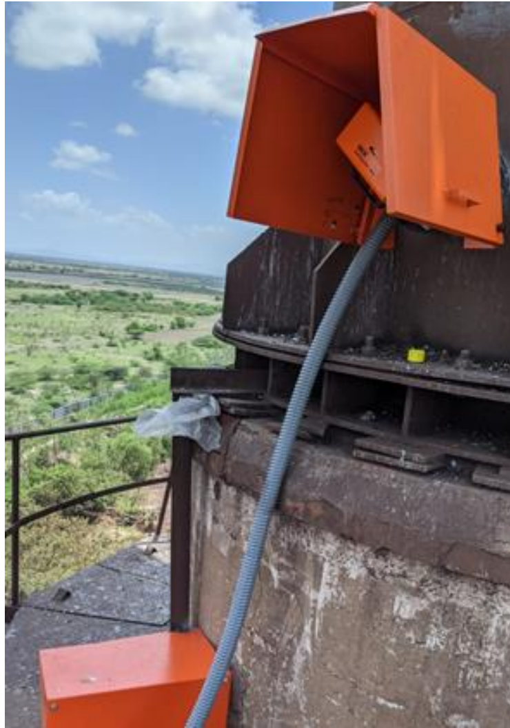
Continuous stack monitoring device Installed at our Rotary Kilns Stack.
