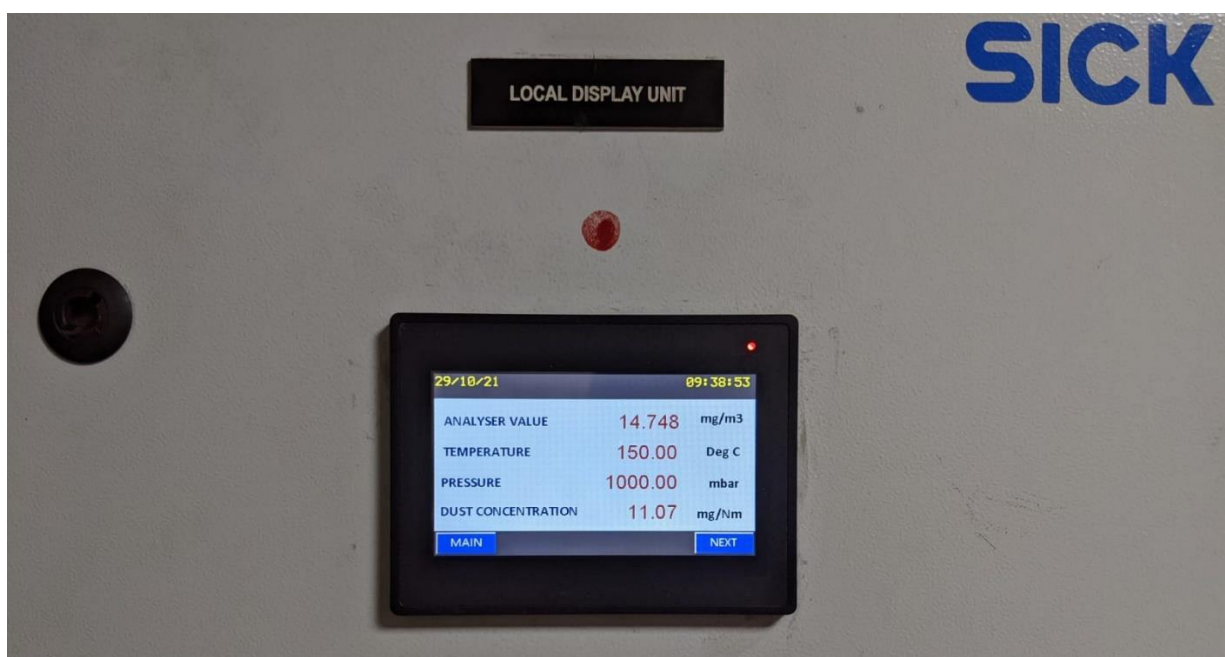
Live Display unit installed at our office.
